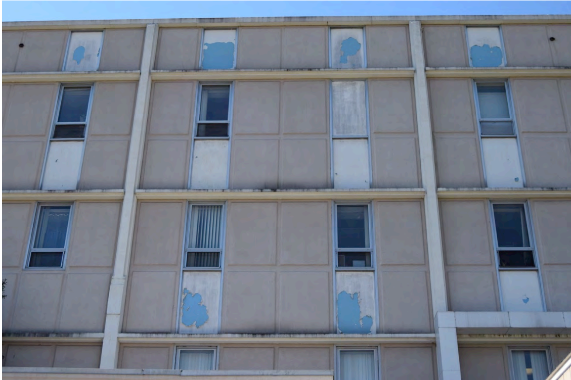
Detail at rear elevation of L. Richardson Memorial Hospital II (GF6065), showing exposed concrete structure and peeling paint at spandrels, view SW.
